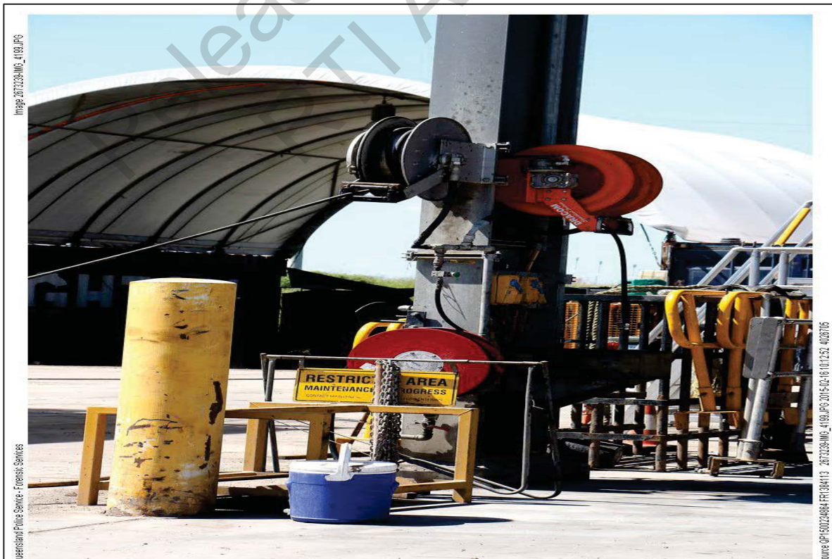
Figure 24: Air supply reticulation supply point (taken by QPS prior to site release).
