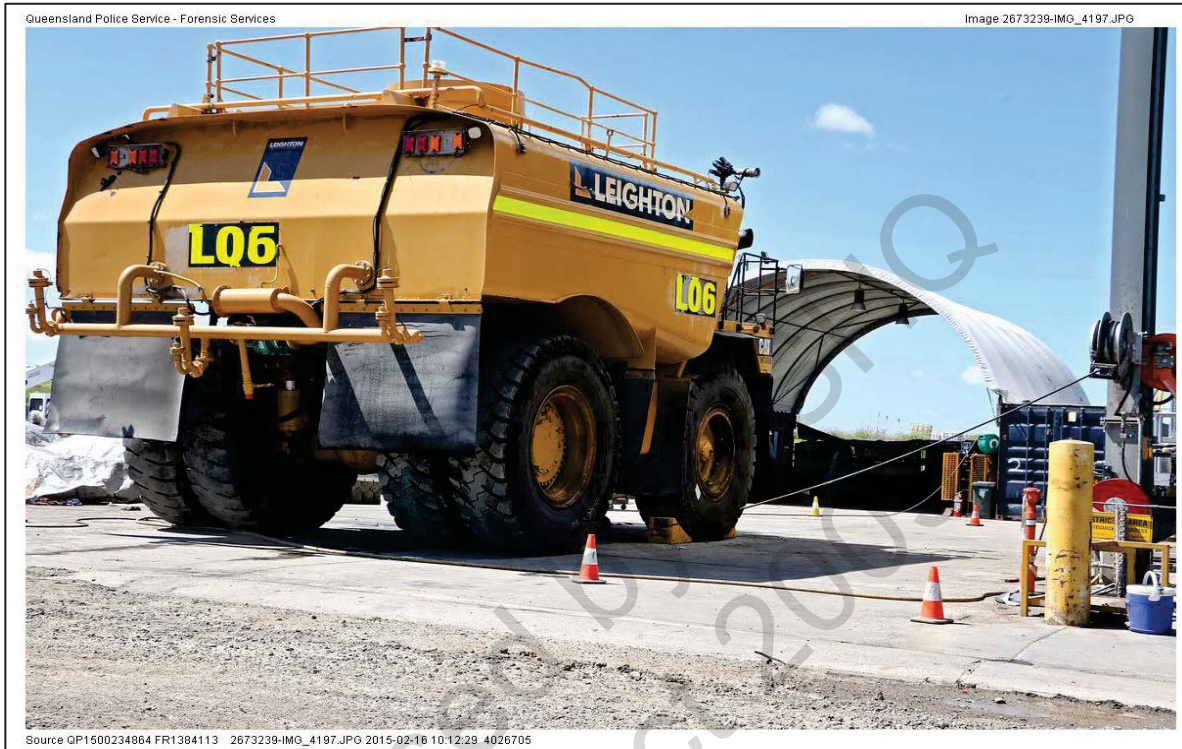
Figure 23: Air supply reticulation supply point (taken by QPS prior to site release).
