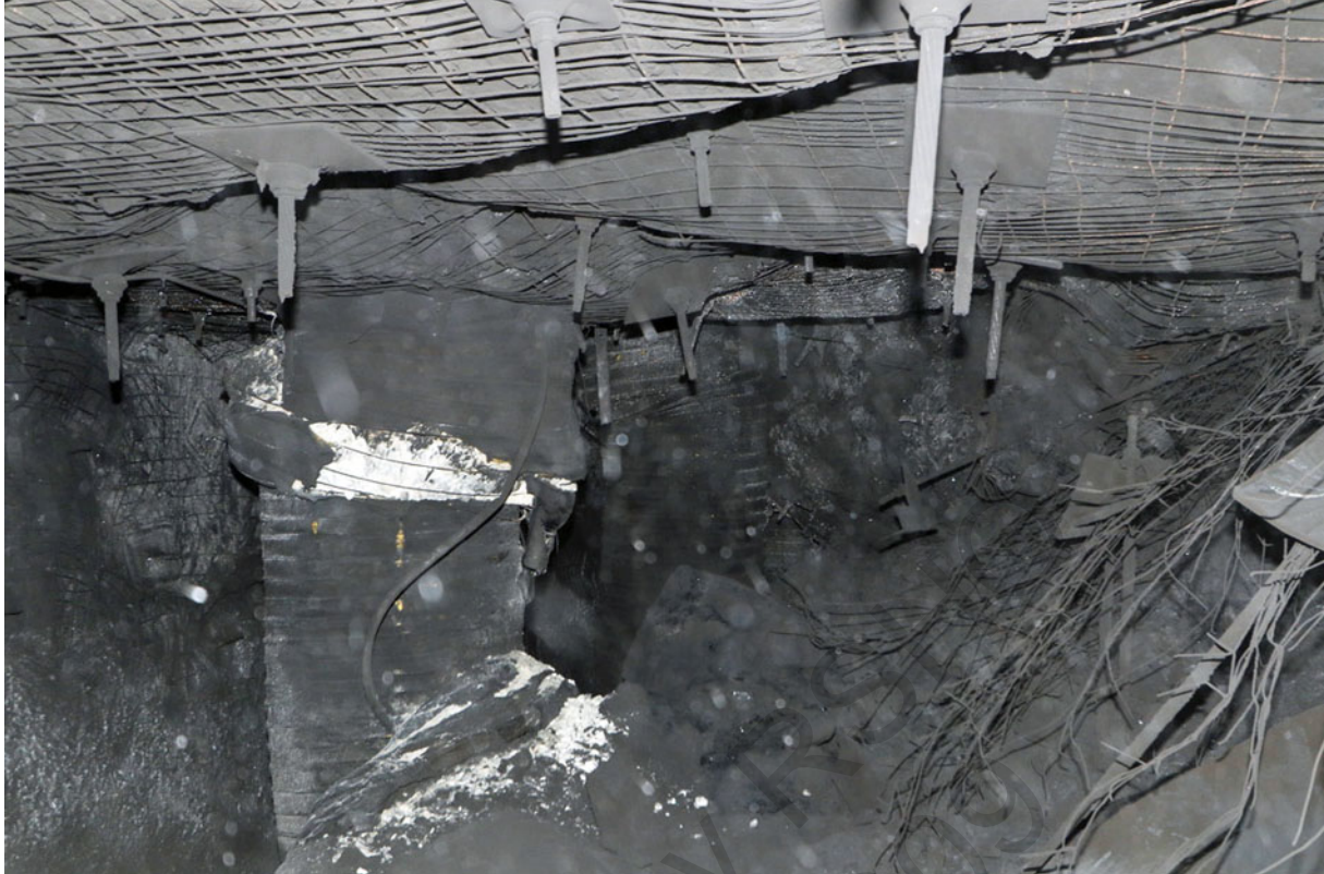
Image 28 Evidence of a roof fall in the goaf to the rear at the Tailgate
